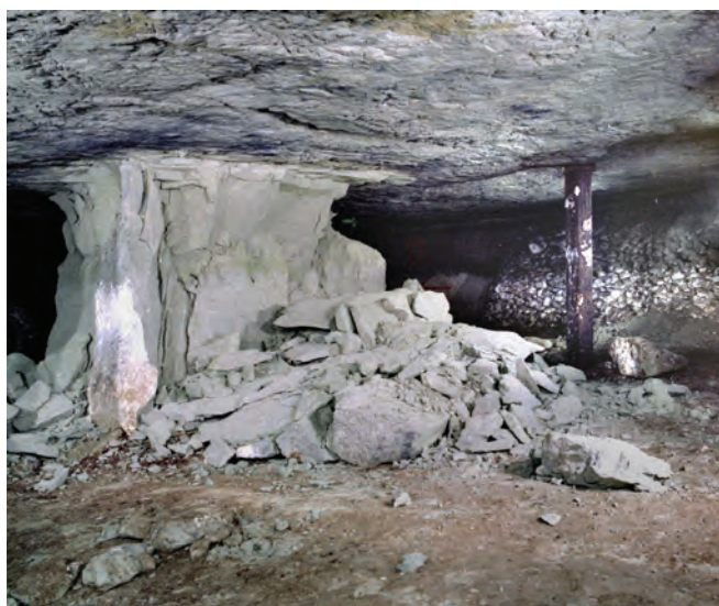
This pillar has been in a state of collapse for 40 years but visitors still always give it a wide berth. Photo Nick Catford
